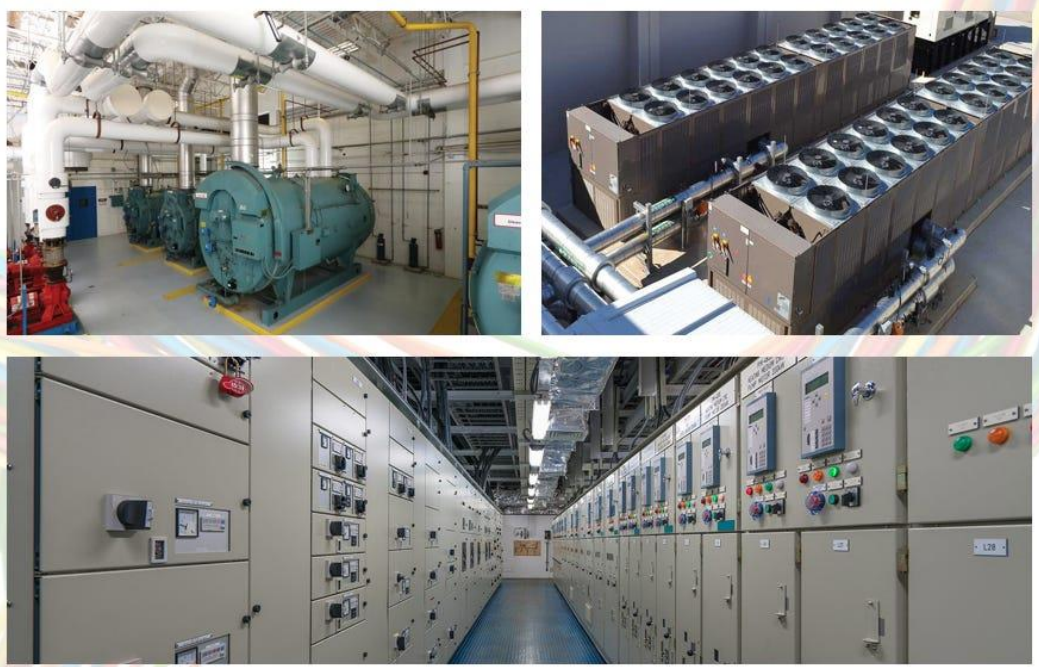
Figure 1: Fire pumps, boilers, AHUs and electrical monitoring (typical MEP)
